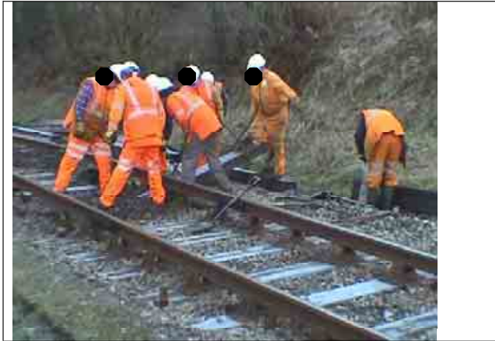
Figure 20. Four workers carry sleeper and place it under the rail. Two workers stand-by in the 4ft to take over lifting the front of the sleeper.
