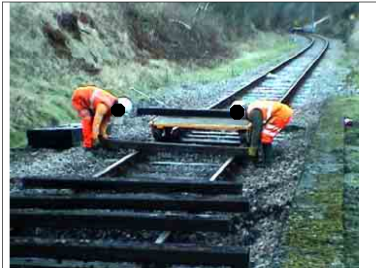
(a) The start of the lift between the rails and the Trolley.
