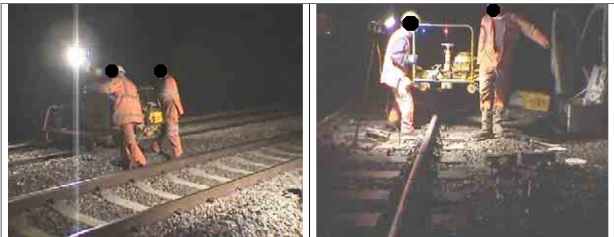
Figure 32. The lifting and carrying of the grinder over the rails. Note that one worker lifts with one arm in both cases.
