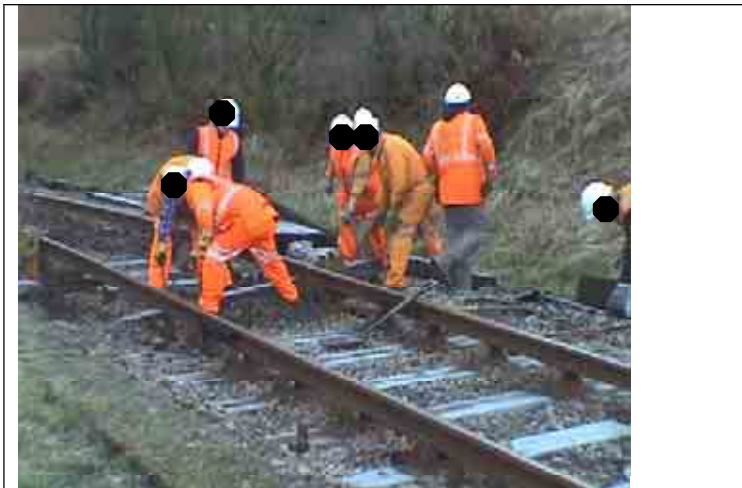
Figure 21. The two workers take over the nips at the front of the sleeper and drag in right through under the 2 nd rail.
