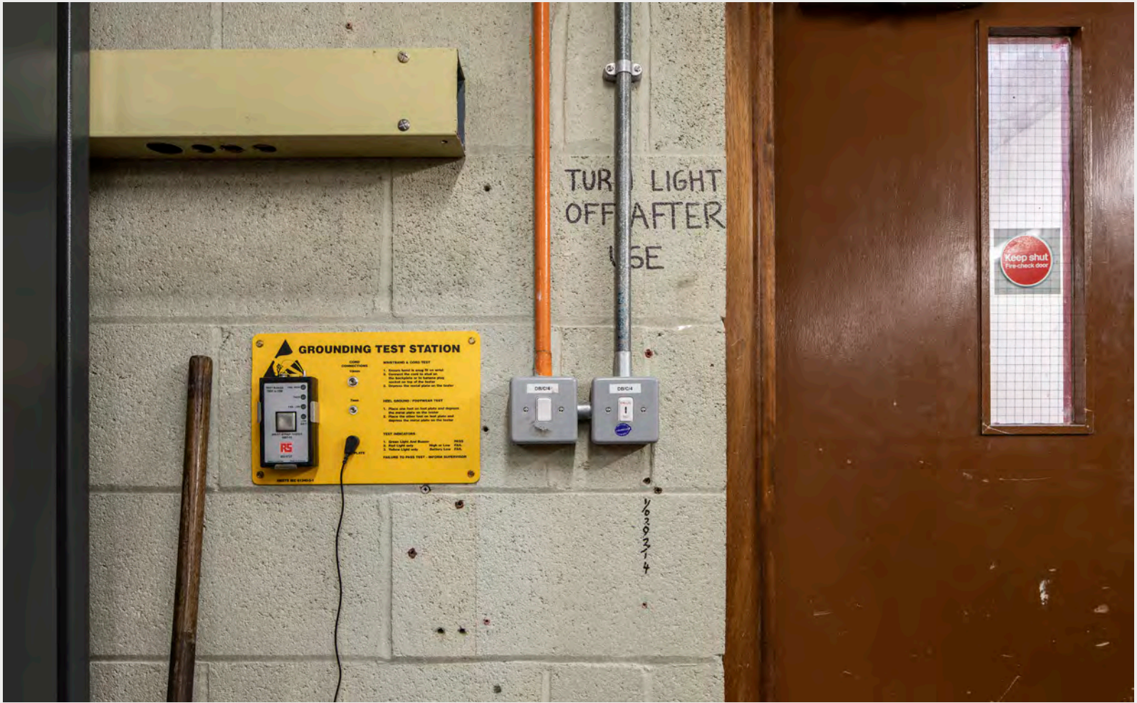
Signalling room, Doncaster. Image © Adelina Iliev.
