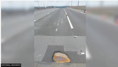
NATIONAL HIGHWAYS | A National Highways spokesperson confirmed a team was deployed to make "emergency repairs" to the road
